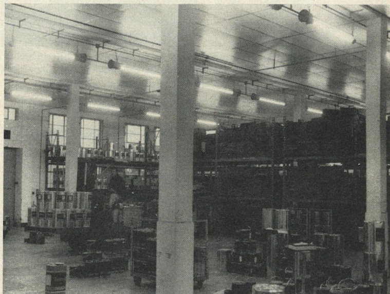
Flameproof fittings in the paint works
